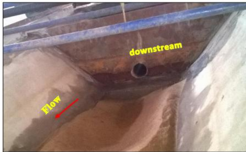
Photo 2. The coverage and its scoured soil basin.
