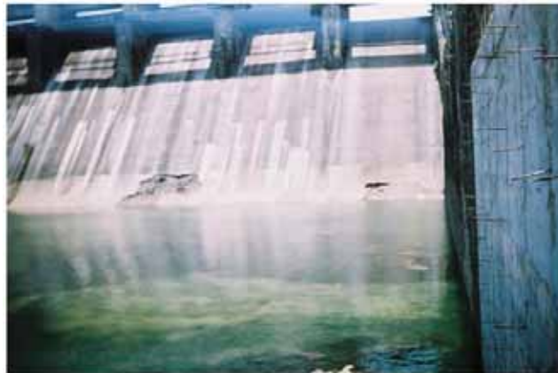
Fig. 2. Photograph showing typical erosion at toe of Pawana dam spillway
