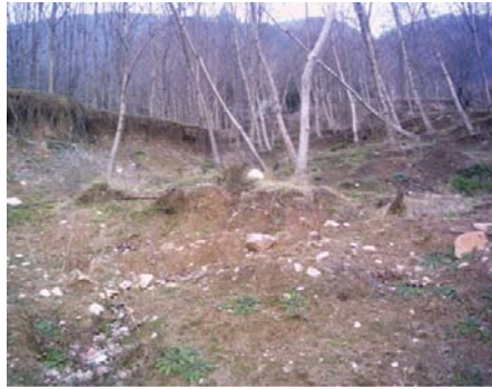
Fig. 4: A view of the active slide at the site – tilting trees and visible roots indicate an active fault in the area.
