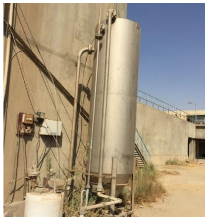
Figure1: Shows Pilot Unit of Dyna Sand.
