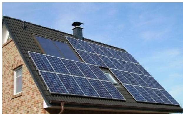
Fig. 4: Fixed solar panels mounted on the roof
